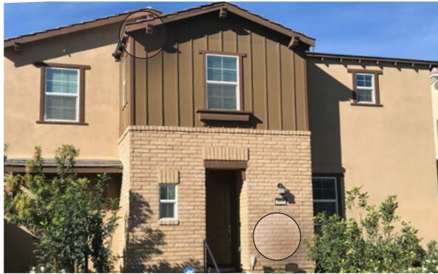
Exposed rafter tails at select locations & brick veneer
