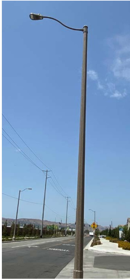
Collector Street Light, Cobra Fixture
